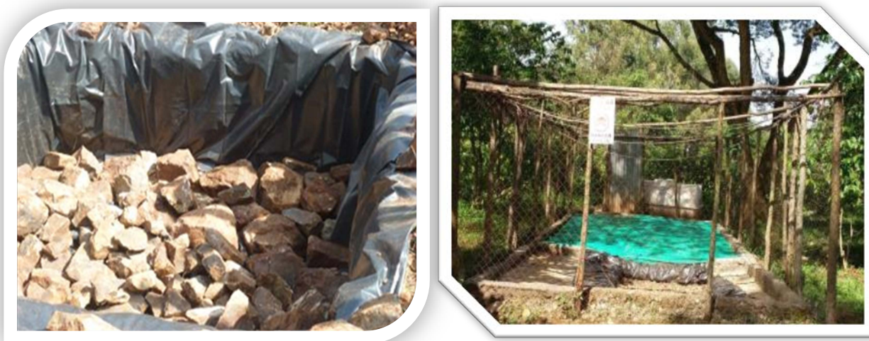
FIGURE 6. PLASTIC SHEET LINING INSTALLED TO PROTECT SIDE LEAKAGE OF EFFLUENT IN KERSA DISTRICT
