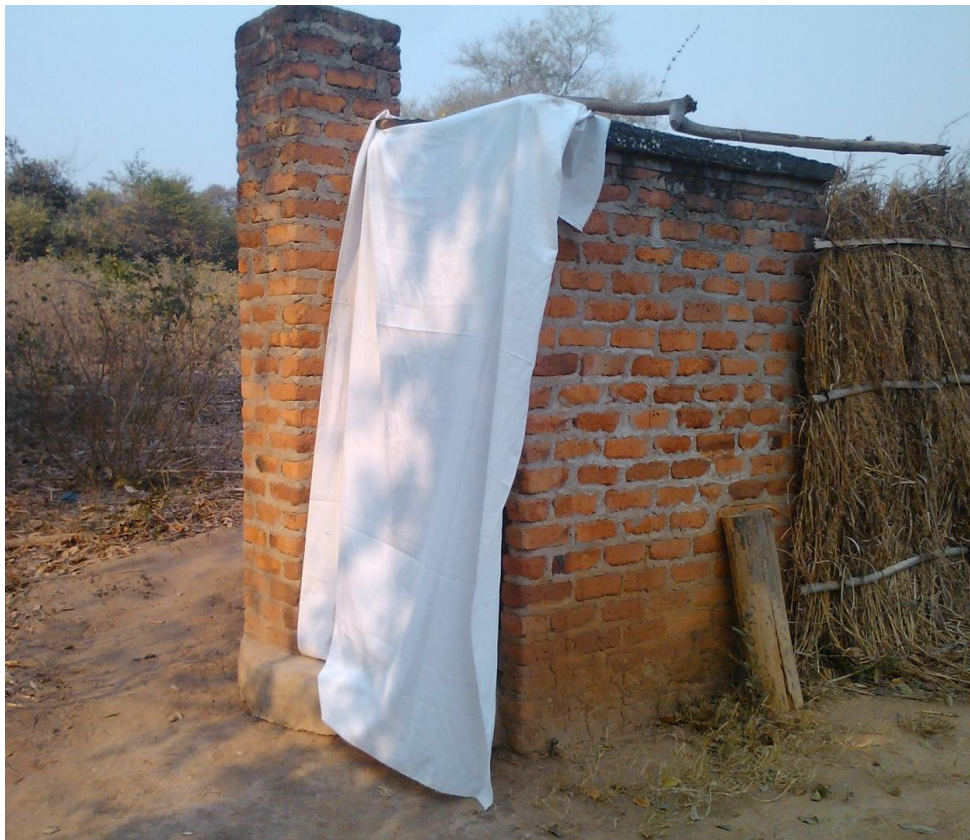
FIGURE 1: WHITE CLOTH COVERING THE ENTRANCE OF A PIT LATRINE FOR PSC, BURMA VALLEY
